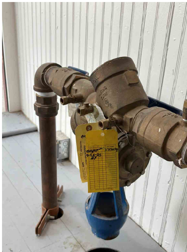
Photo-20 Interior 5 side floor 1 RPZ backflow preventer.
