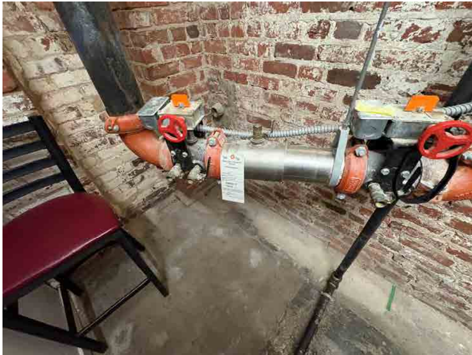
Photo-18 Interior basement fire sprinkler controls
